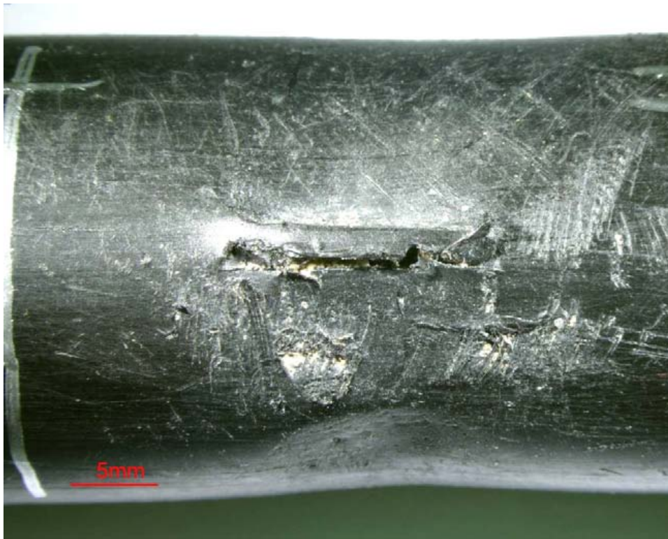
Figure 24. Failure at a squeeze-off – Bakersfield.
